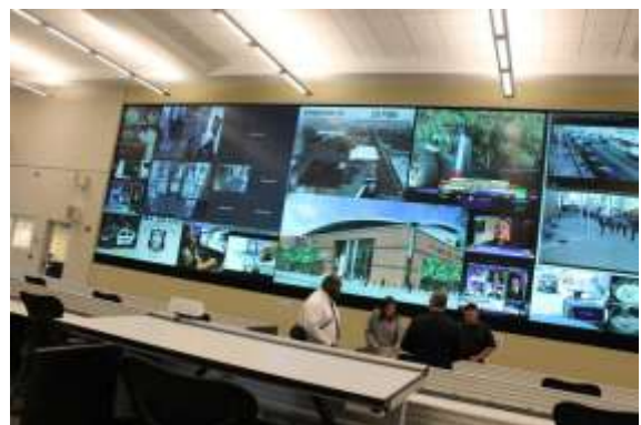
Command Center monitors city video feeds
