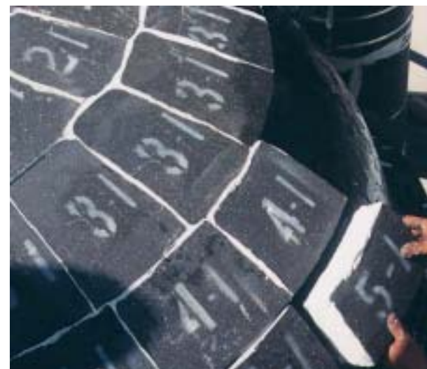
Pamrod HATS were installed while this cryogenic tank was in operation.
