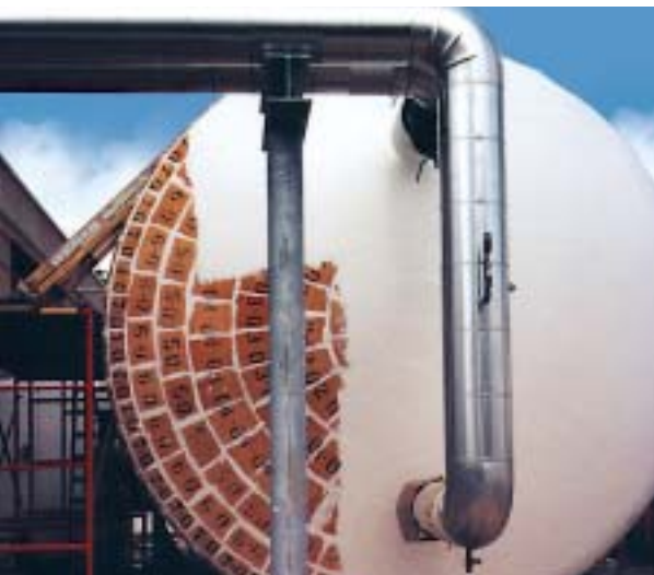
Field cutting insulation for this storage tank would not appear nearly as precise as the Pamrod HATS installed here.
