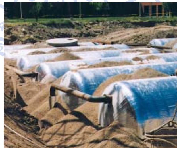
These buried hot and chilled water tanks were insulated with Pamrod HATS for trouble-free performance.
